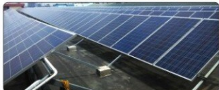
1 MW Rooftop Solar Power Plant at IOCL Panipat.
